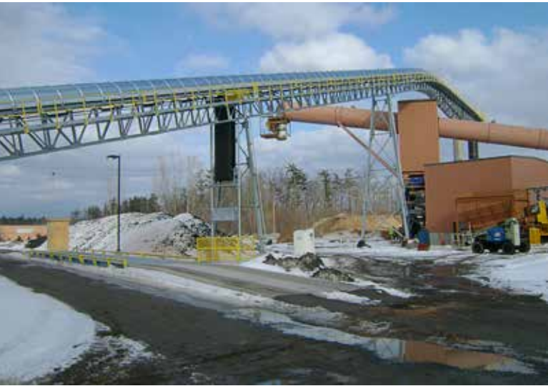
The long conveyor that passes across the Fort Drum access road and delivers fuel to the wood yard on the other side.
