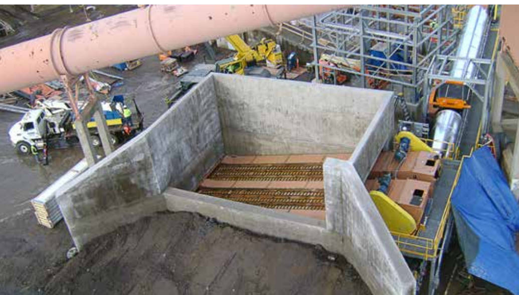
The reclaim area with drag-chain reclaimers (center) and the transfer belt that leads to the legacy boiler feed system (top right).
