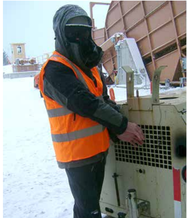
A ProcessBarron engineer warms his hands during the cold, outdoor equipment installation at the Fort Drum site in January 2013.
